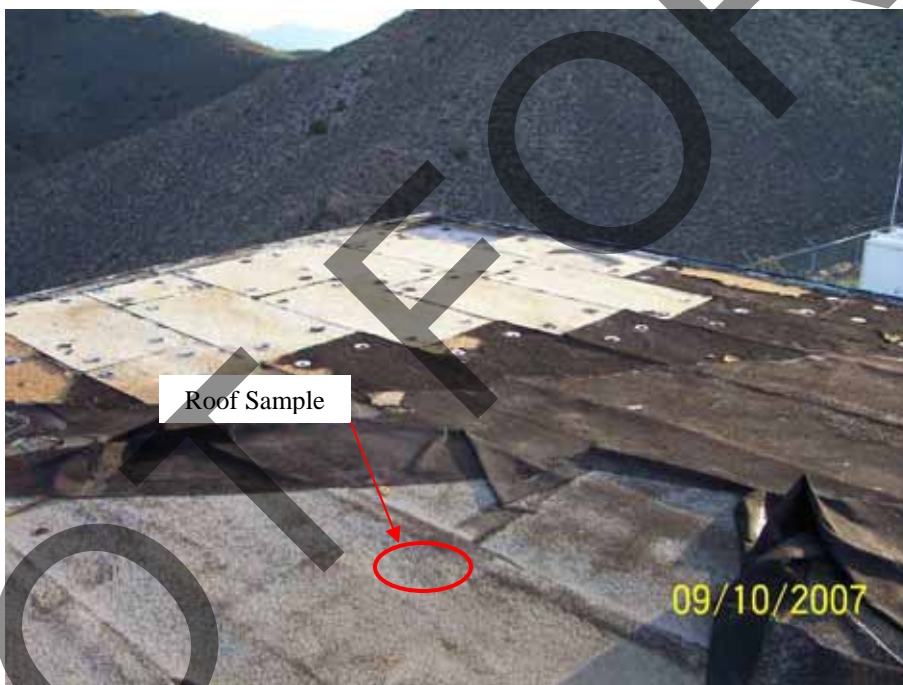
6. View of the damaged roof in the southwest portion of the Subject Property building roof.
