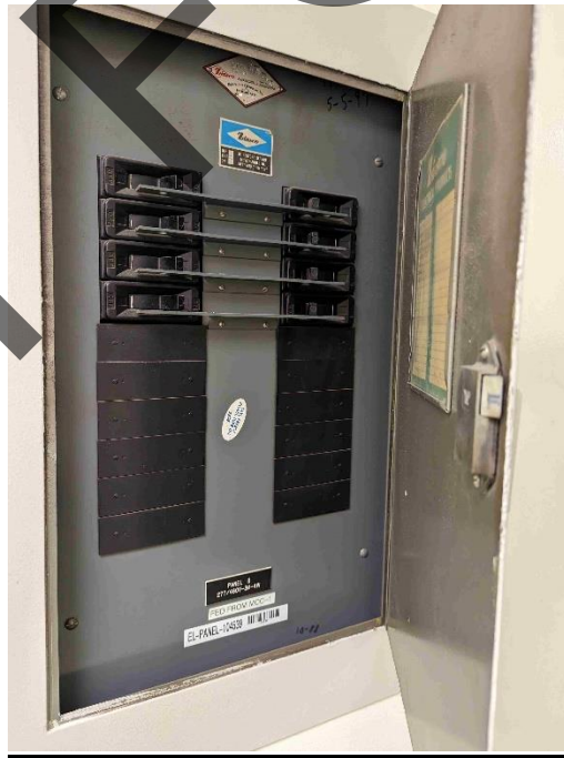
Detail 1/1 st – Electrical Circuit Breaker Panel “B” on the First (1 st ) Floor
