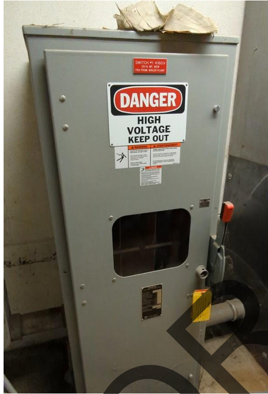
Detail 3/BM – Electrical High Voltage Switch in the Basement (BM)
