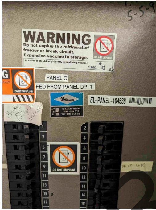
Detail 2/1 st – Electrical Circuit Breaker Panel “C” on the First (1 st ) Floor
