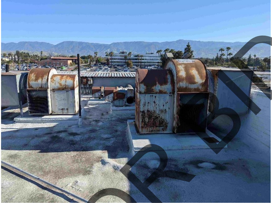
Detail 1/ROOF – Mechanical Equipment on the Roof
