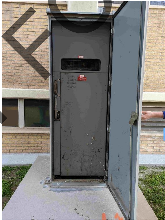
Detail 1/EXT – Empty Electrical High Voltage Cabinet
