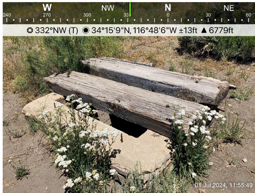
Photograph 13. Abandoned mineshaft containing standing water at a depth of 10 to 15 feet at the time of the field investigation facing northwest.
