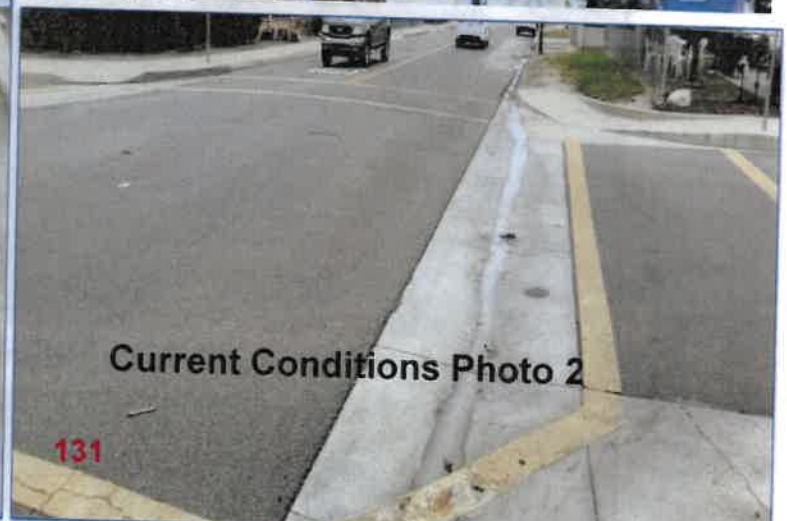
No ADA Curb Ramp, Existing Conditions Photo 1
