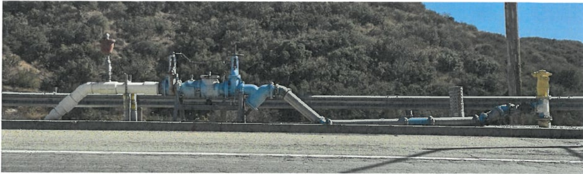
Figure 28 Water connection OSY (Photo provided by Bergman Development Services)
