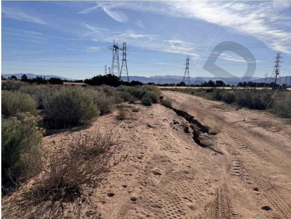
Photograph No. 2, Current alignment conditions at BH-04 on Rodeo Road, view to east.
