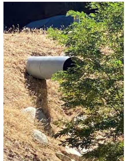
Figure 13 Extreme Stormdrain Outlet Erosion
