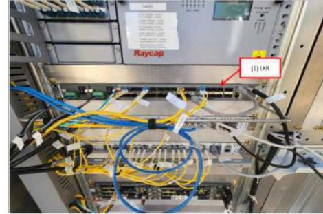
3 VZW IXR PANEL INSIDE EQPT CABINET
