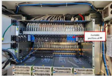
1 VZW EQUIPMENT CABINET FRONT VIEW
