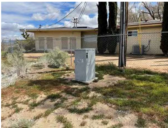
Photo #23 View of pad-mounted transformer on northwestern portion of complex.
