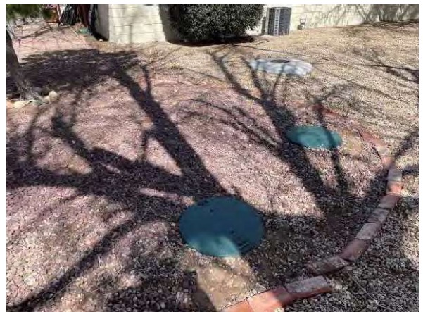
Photo #6 View of subgrade grease trap system, located in the central portion of the complex to the north of the kitchen area.
