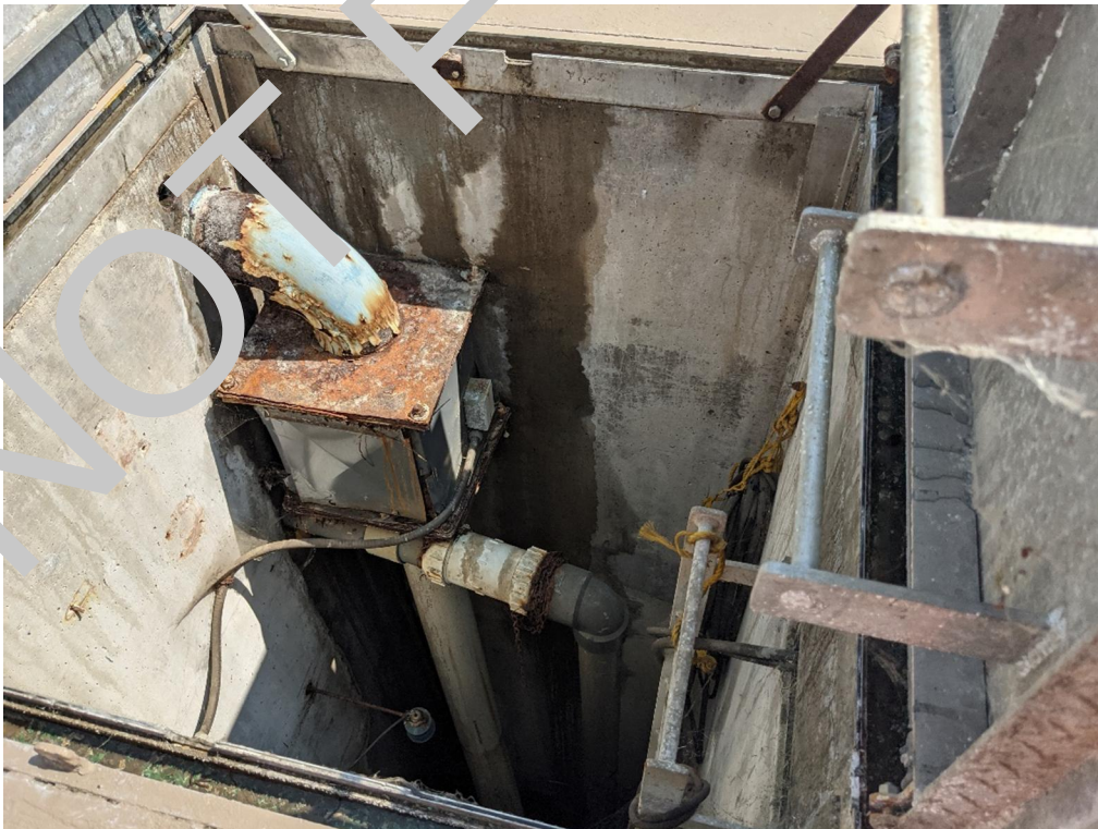
Wet Well Hatch and Riser
