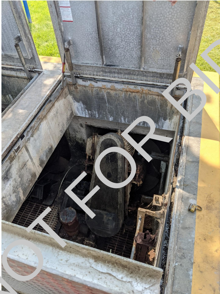
Discharge Structure and Screw Pumps
