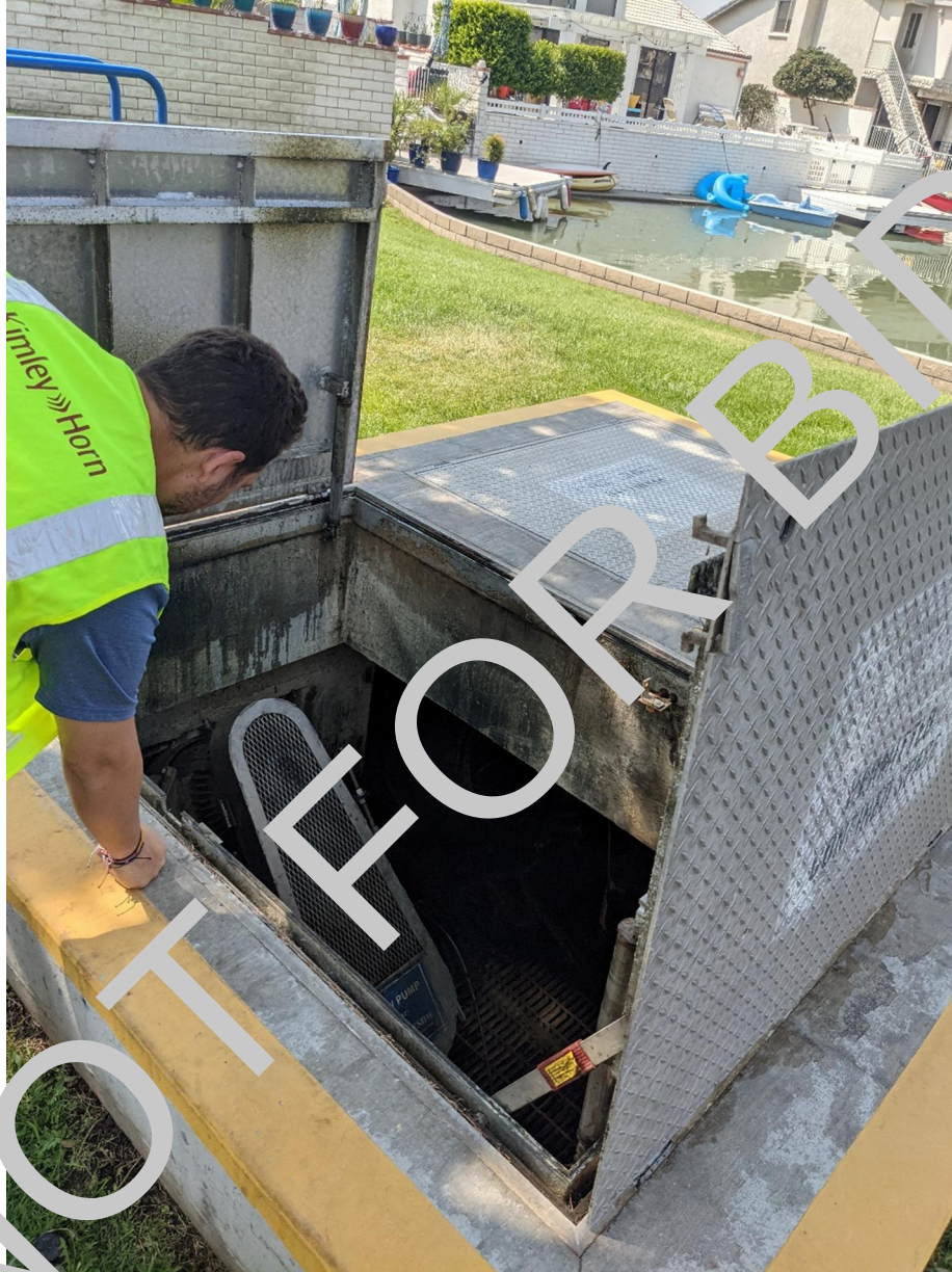
Discharge Structure and Screw Pump
