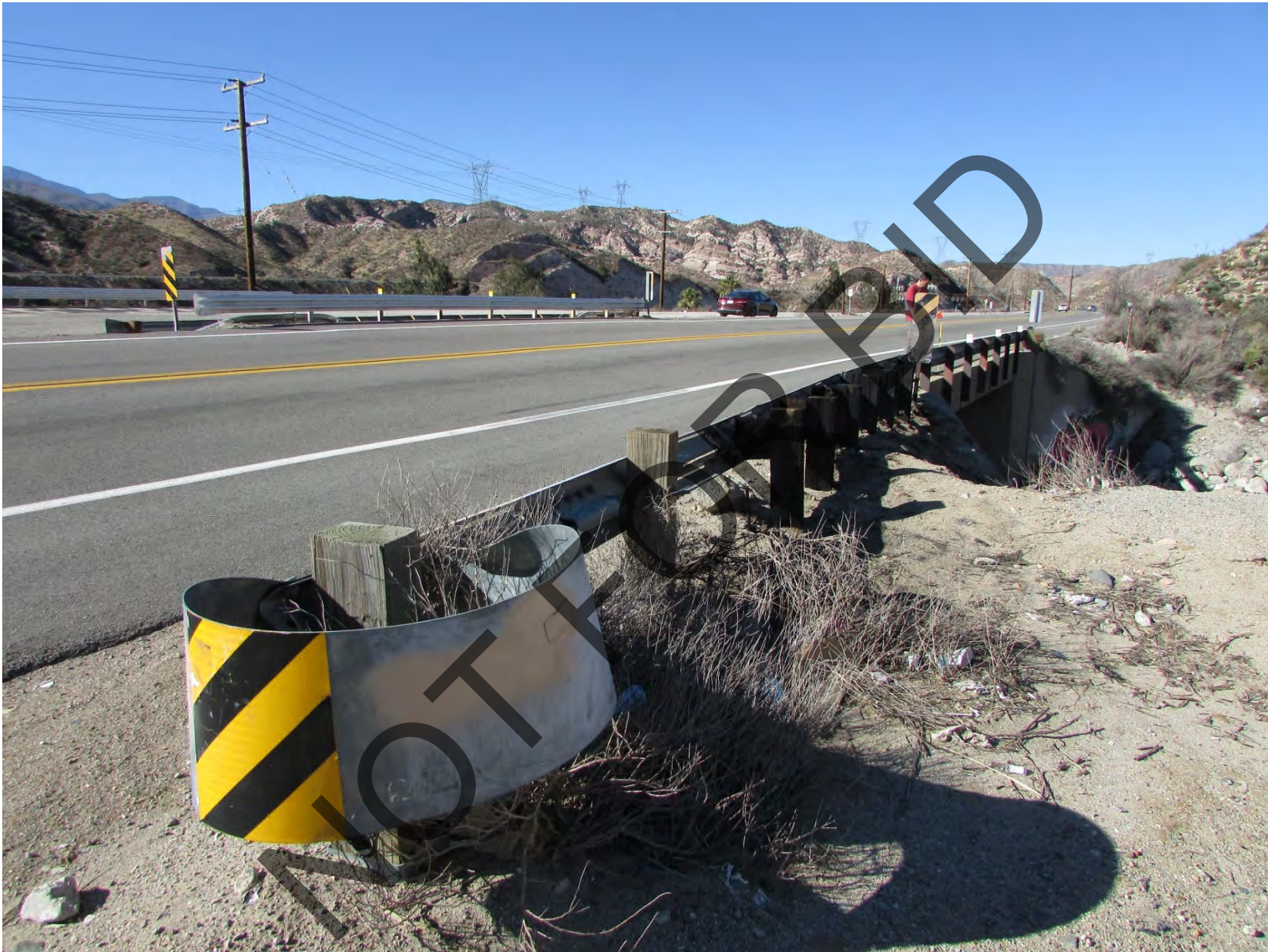
9.6) Devore Area: Cajon Blvd_ Railing at Bridge
