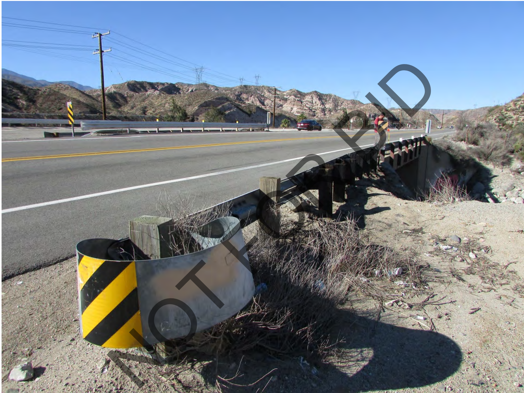
9.6) Devore Area: Cajon Blvd_ Railing at Bridge
