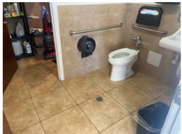
Photo #18 Typical view of interior floor drains located in the restrooms on site.
