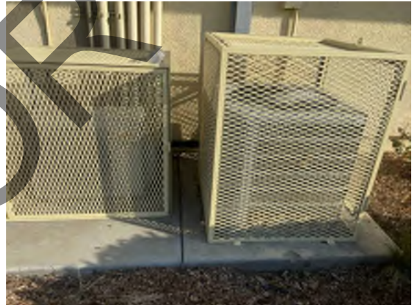
Photo #16 View of the HVAC systems located near the residential duplexes.
