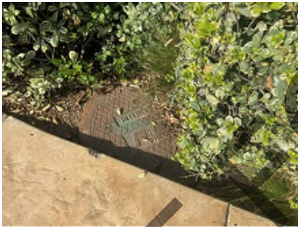
Photo #21 View of a grease trap located on the western portion of the site associated with the kitchen.
