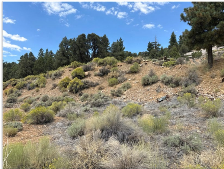
Photo 18. Overview of Locus 2 and Feat-5 (metal pipe), and the collapsed hillside. View towards northwest.
