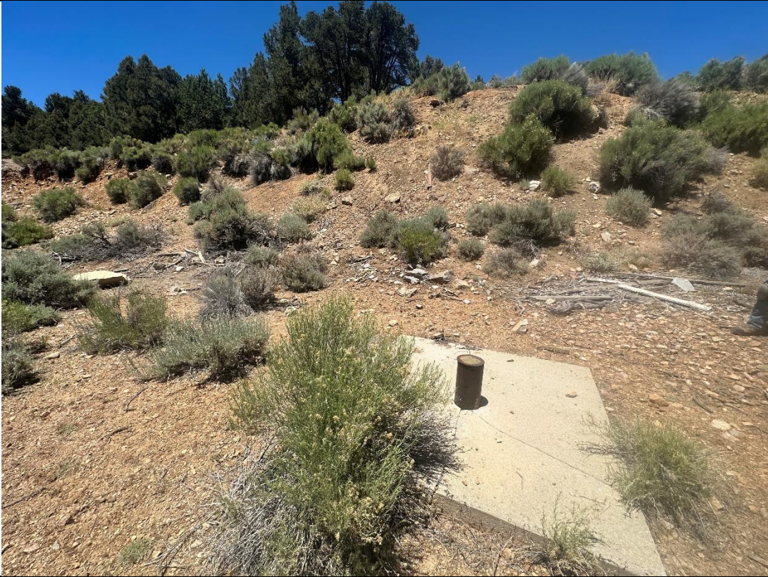
Photograph: 9 Ventilation shaft located directly below the production shaft to the south.
