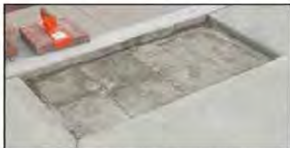
8) Allow concrete to cure. Use the following guidelines based on installation method. Note: If using wet set, do not allow concrete to cure.
