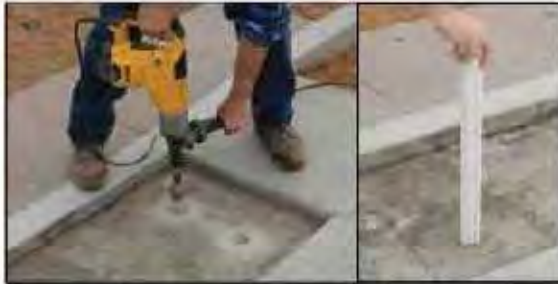
Step #1 - Sand Set Installation - Create weep holes for drainage. Core drill hole once concrete has set or, while concrete is still wet, make a hole with pipe.
