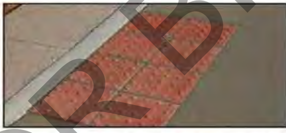
Step #4 - Thin Set Installation - Grout all joints with an exterior based grout or caulk. Complete.
