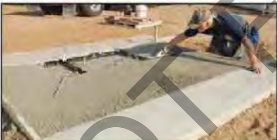
5) Pour concrete into and around frame work. Level concrete and bull float area.
