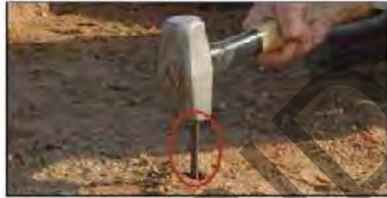
2) Drive in rebar to the approximate height to receive Wausau Tile's block out frame. The frame work has small feet to help locate where rebar should be located.
