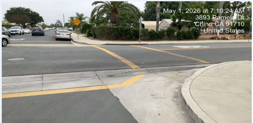
Photo 2. Curb return at the school entrance — no truncated dome warnings or ADA-compliant ramp at this corner.
