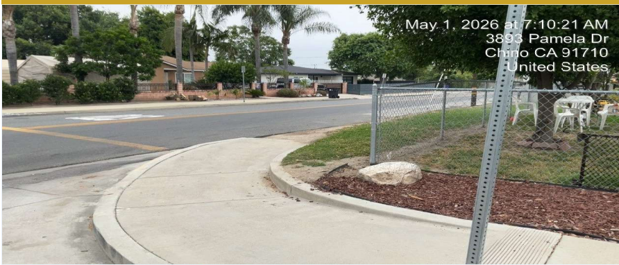
Photo 6. Curb return on Pamela Dr near the school driveway — no ADA ramp serves this corner.
