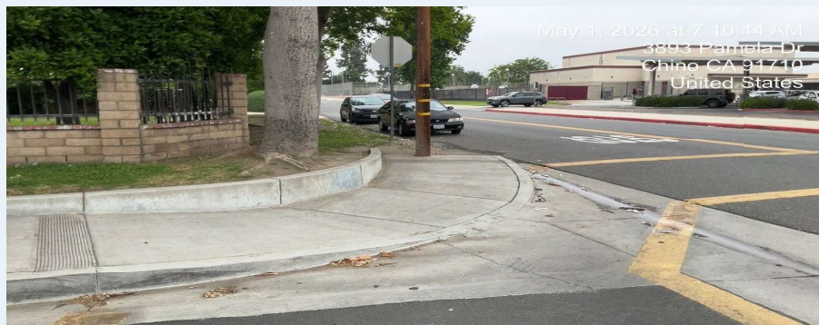
Photo 3. Faded standard crosswalk striping at the school crossing — no high-visibility (continental) markings.
