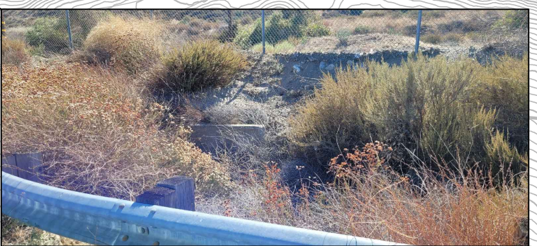
LOCATION #5 OBSERVATION #5: EXISTING DRAINAGE FACILITIES ARE LACK OF MAINTENANCE
