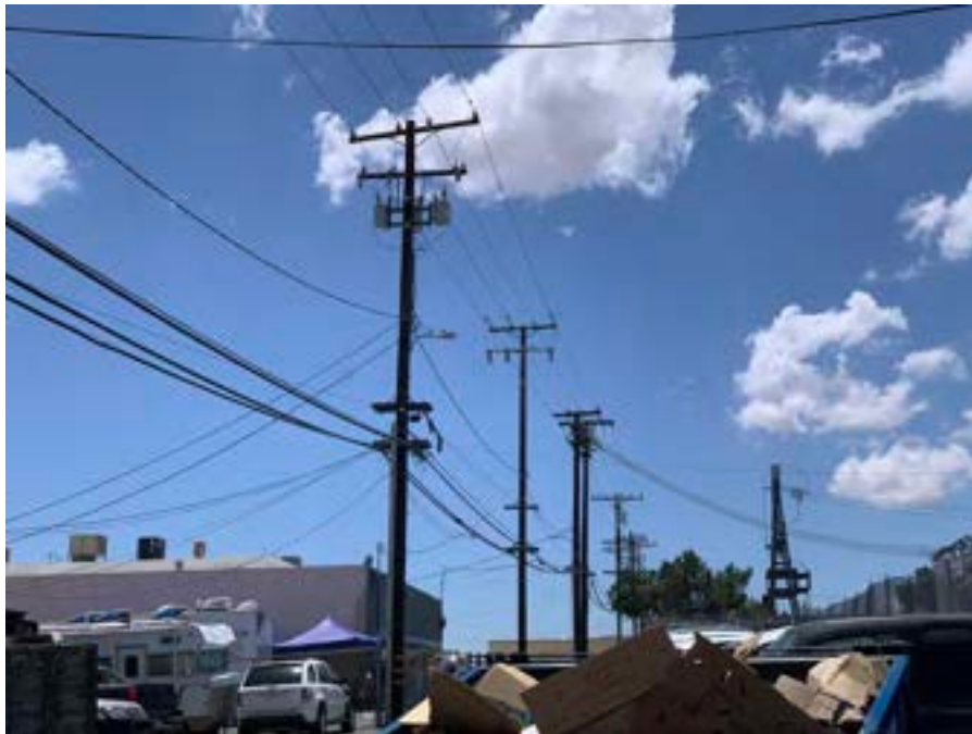
Site Photograph 12 – PMT located southwest of site
