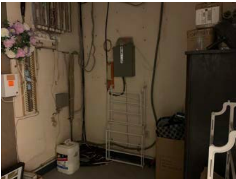
Site Photograph 26 – Interior - Communications equipment
