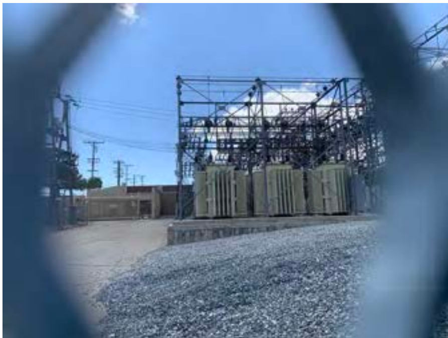
Site Photograph 10 – Looking southwest away from site into SCE substation
