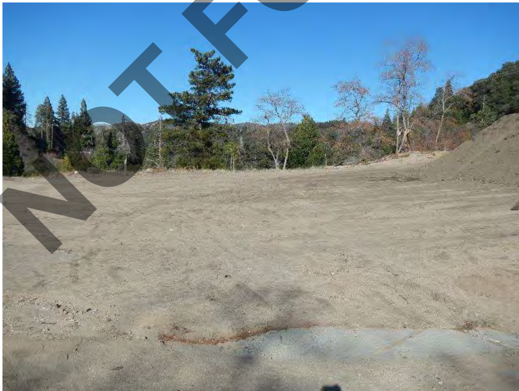
Photograph 12: View of the sediment storage area, Camp Switzerland, in the northern portion of the project site.
