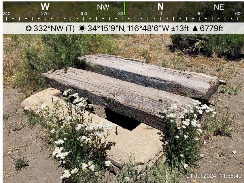
Photo 13. Abandoned mineshaft containing standing water at a depth of 10 to 15 feet at the time of the field investigation, facing northwest.
